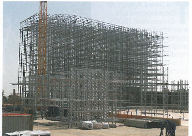
Universal Storage Systems new clad rack warehouse for UTi Pharma under construction.
