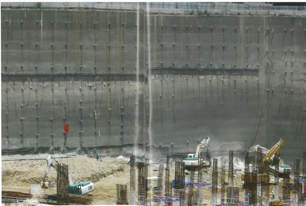
North western corner of the site where the excavation depth reached 32 m.
