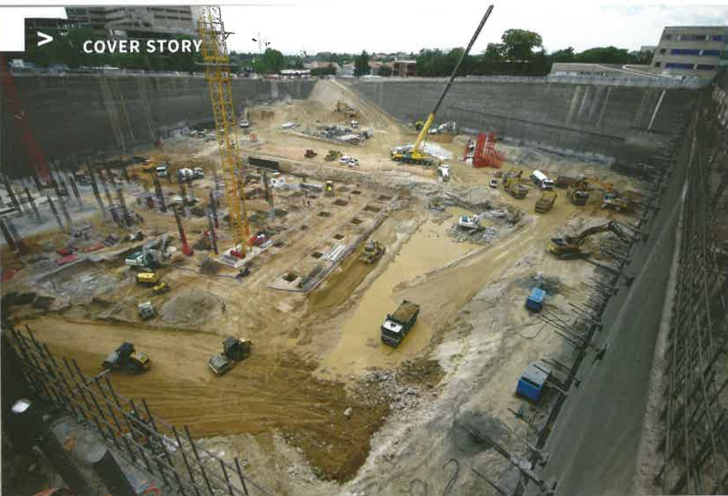
An overall view of the site as seen from the north western corner.
