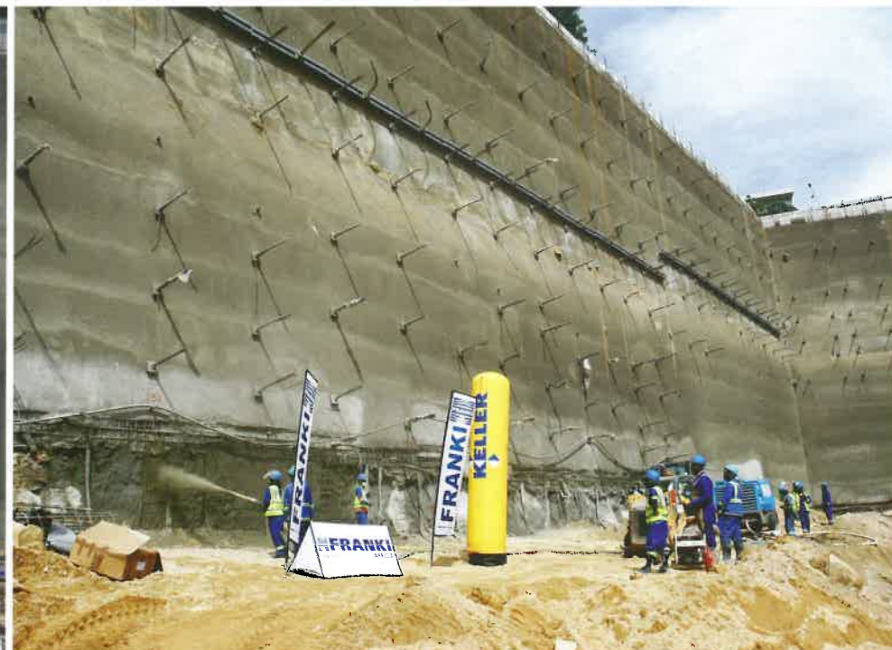
Gunite being applied to the trimmed face along the southern portion of the site.
