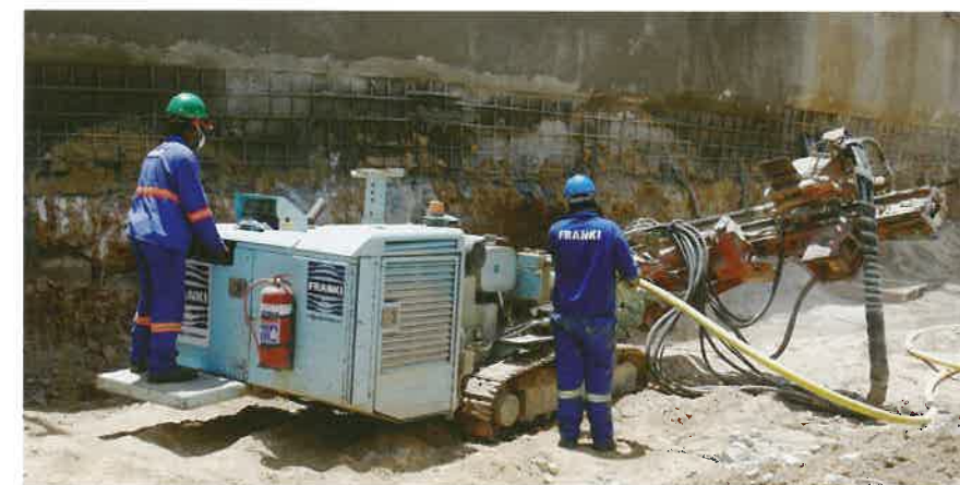
Drilling for the installation of the strand anchors. In instances, 25 m long anchors were installed.
